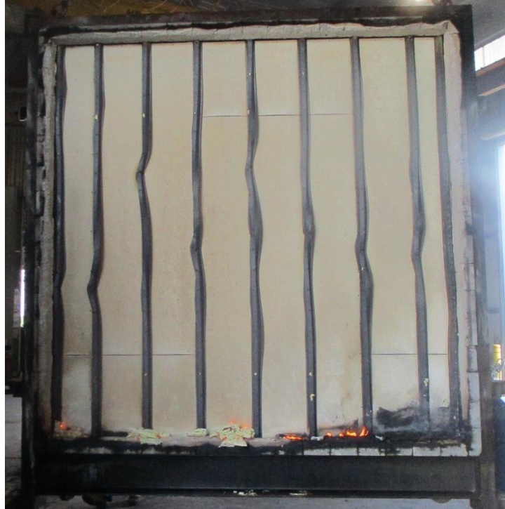
Photo No. 51 Exterior Exposure - Exposed Face – (Post-Fire Resistance Retest Period)
