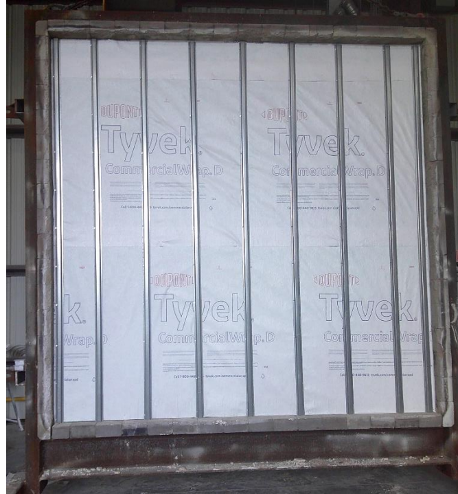
Photo No. 8 Completed installation of 1-1/2-in. deep hat channels spaced 16-in. on-center Interior Exposure
