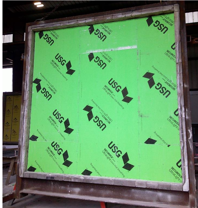
Photo No. 31 Completed face layer of Exterior GWB on exposed face Exterior Exposure
