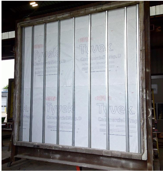
Photo No. 33 Completed installation of 1-1/2-in. deep hat channels spaced 16-in. on-center Exterior Exposure
