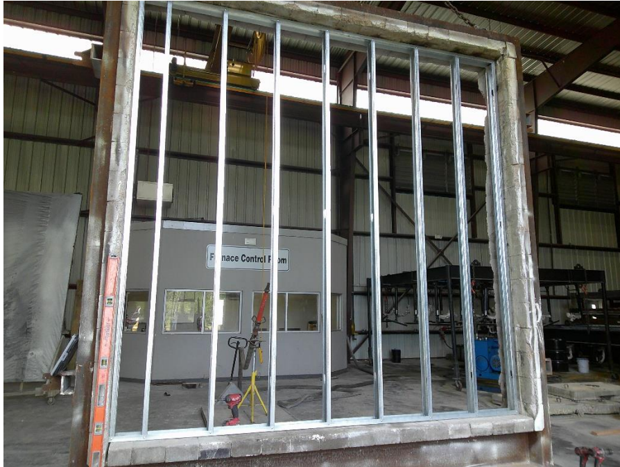
Photo No. 27 Completed framing of base wall assembly. 20-ga. EQ., 3-5/8-in. steel studs spaced 16-in. on-center Exterior Exposure
