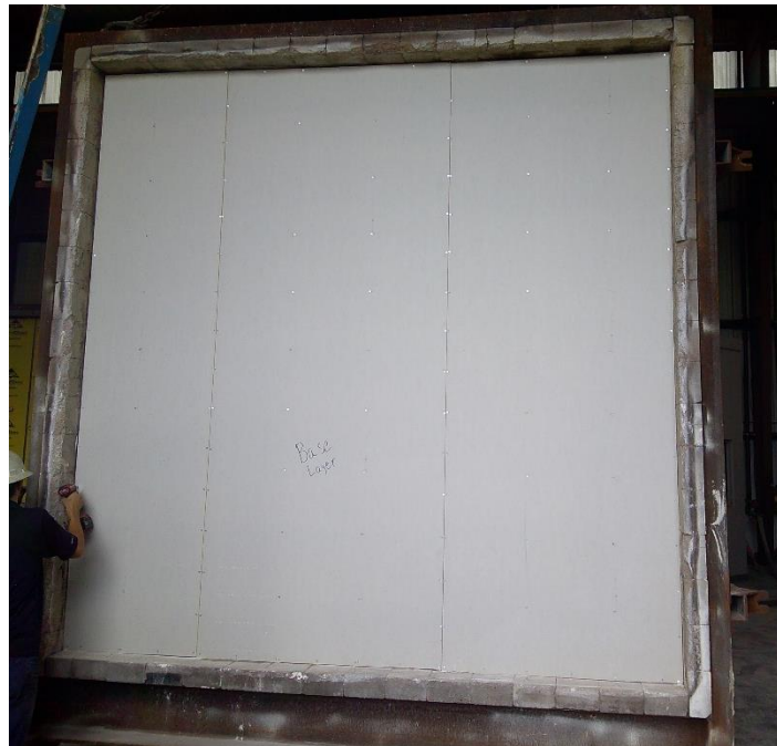
Photo No. 30 Completed base layer of GWB on exposed face Exterior Exposure
