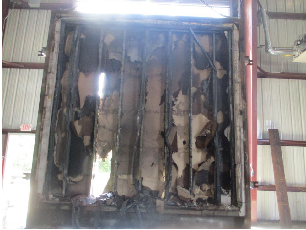
Photo No. 43 Exterior Exposure - Unexposed face - (Post-Hose Stream Application)
