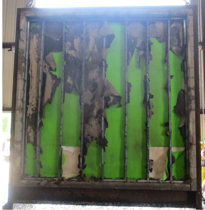
Photo No. 23 Interior Exposure - Exposed face – (Post-Hose Stream Application)
