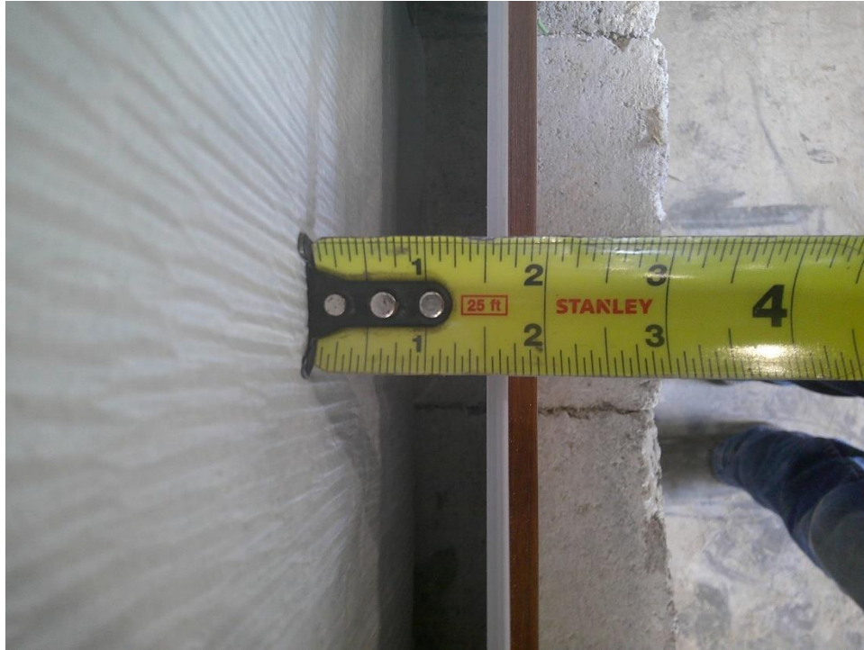
Photo No. 9 Air Gap dimensional detail between WRB and backside of exterior cladding Interior Exposure
