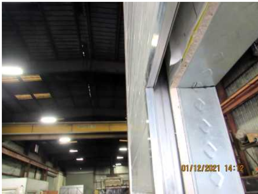
Photo No. 2 Window Trim Installation Sans Window Flashing
